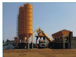
Concrete Batching Plant
