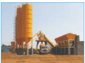
Concrete Batching Plant
