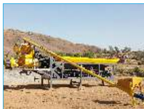
Mobile Batching Plant
